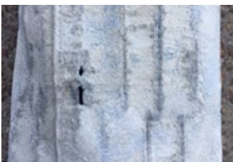
Before – Frequent Failed Filter Bags
