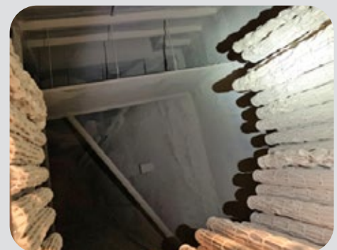
AFTER – PrimaFlow™ implementation resulted in significantly improved baghouse performance
