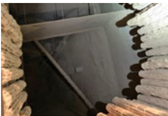
After – SOLAFT® StarBag™ implementation resulted in significantly improved baghouse performance
