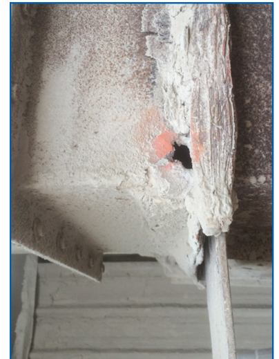
Expansion Joint Leakage
