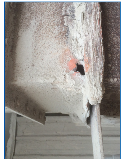
Expansion Joint Leakage
