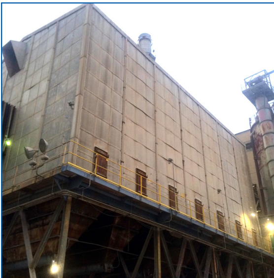
Reverse-Air Kiln Baghouse
